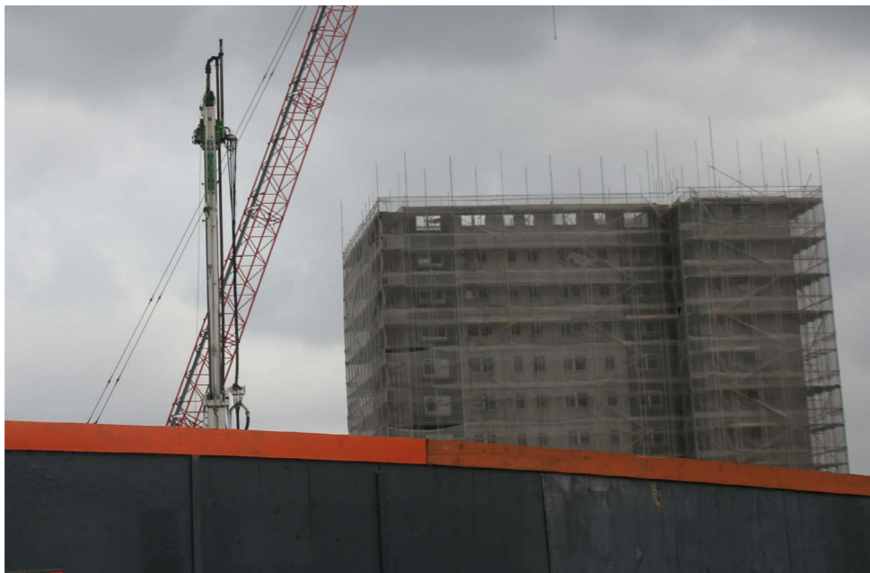
One of several photos I took from the same spot to document the demolition process
