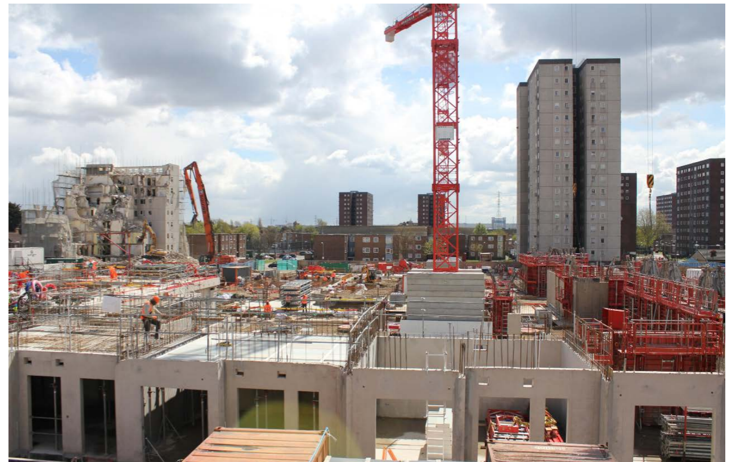
Photo taken by me, April 2016. The view from the construction site window, showing an old block alongside the new build, as another tower is pulled down.
